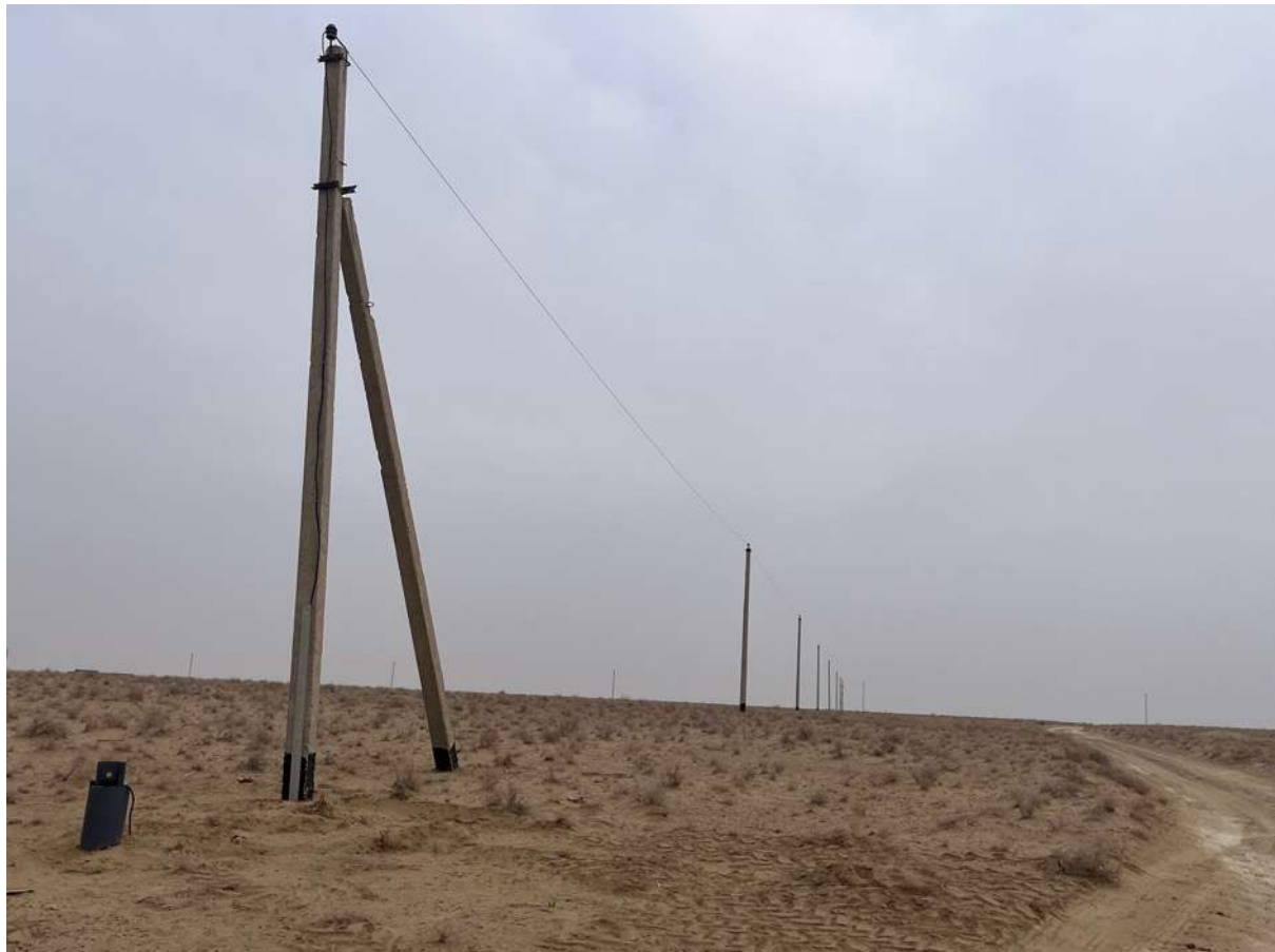
Figure 10-2 Powerline within the Site
