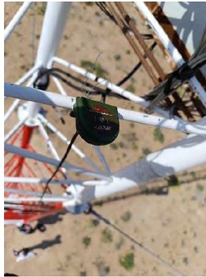
BD03 (North mast - 10 meters)
