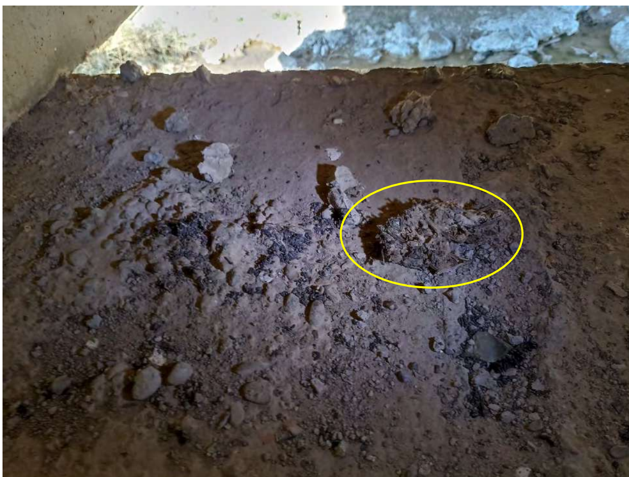
Figure 22. Bat droppings and dead bats (yellow oval) under a concrete bridge (location 8 in Table 2,
