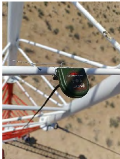
BD07 (South mast - 10 meters)
