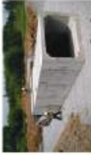
RC Stormwater Drain
