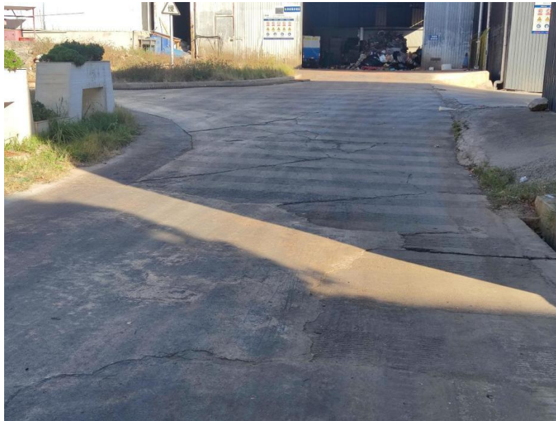
Fig. 6 Concrete floor with cracks in the domestic waste temporary storage area
