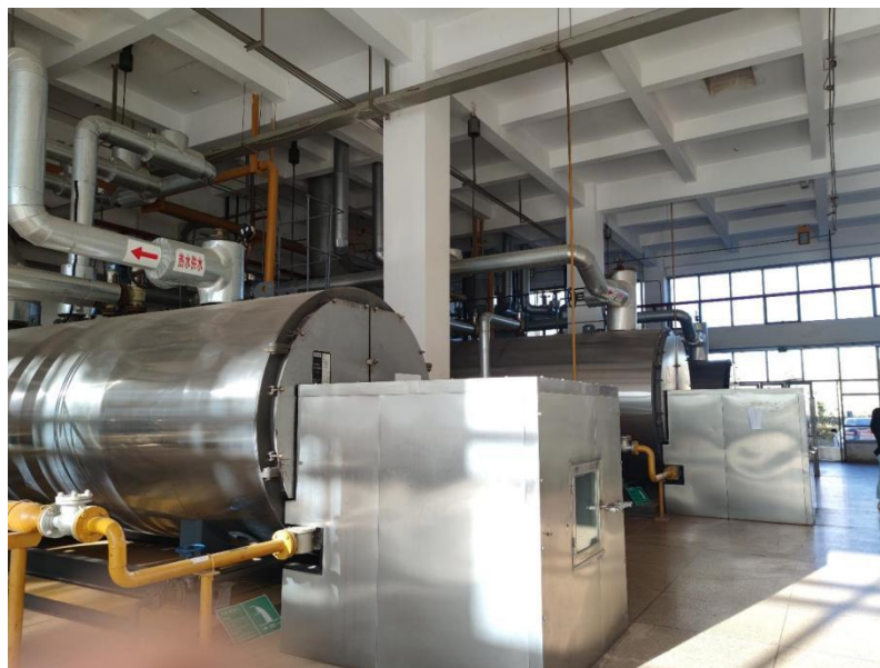
Fig. 10 Gas Boilers at Power Energy Center
