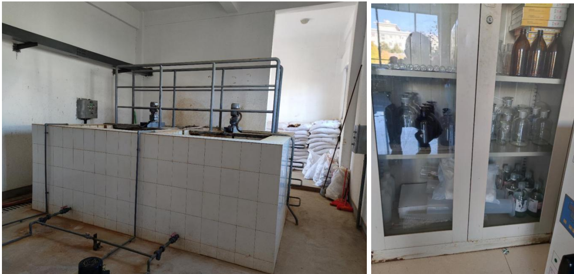
Fig. 2 Dosing system and chemical storage for wastewater treatment
