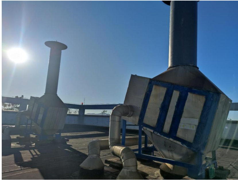
Fig. 11 Gas boiler stack
