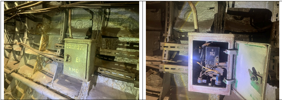
Figure 4: Trackside Signaling Junction/control Boxes
