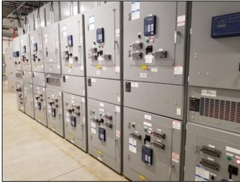
Figure 3-10 Indicative implementation of MV switchgear
