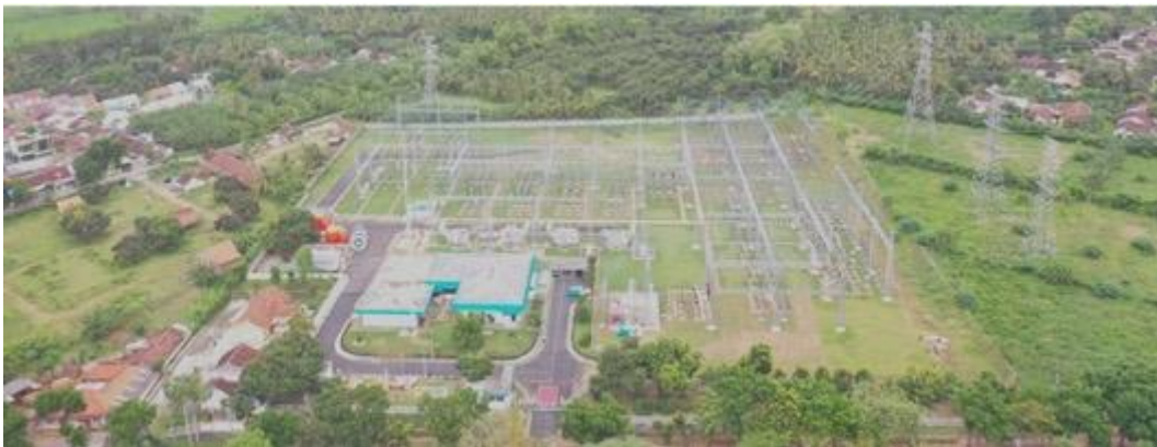
Figure 3-11 Aerial view of existing Banyuwangi Substation
