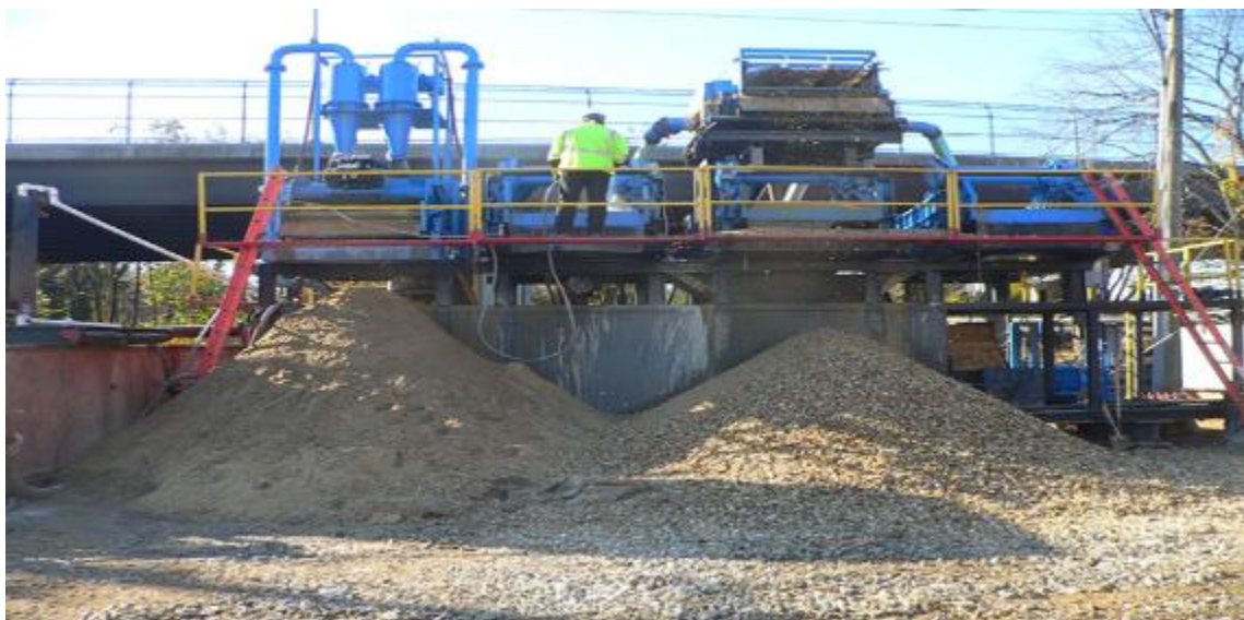
Figure 3-8: Slurry Separation Plant
