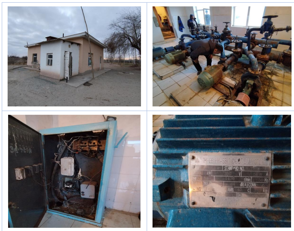
Figure 7: The pumping station in the Sh. Rashidov water intake facility located in Turtkul district
