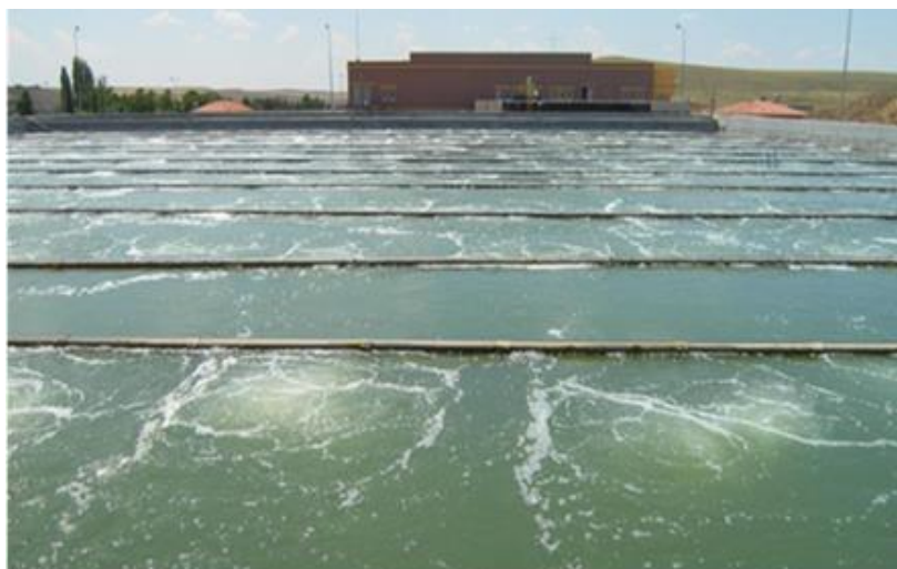
Figure 19: Example of aeration tanks
