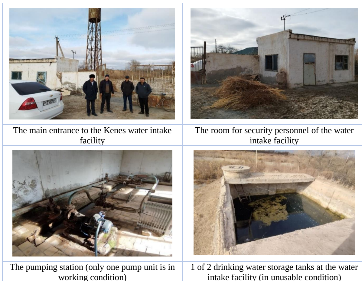
Figure 9: Kenes water intake facility and the pumping station located in Turtkul district
