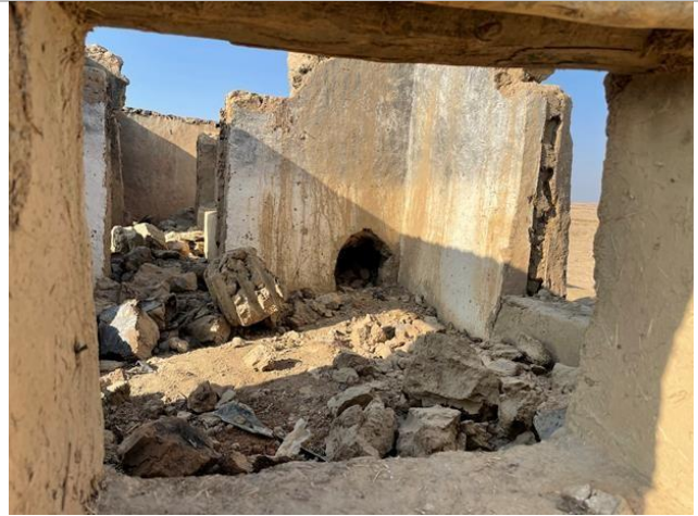
Figure 6-2 Destroyed building built by leaseholder 4 in the Solar PV Area
