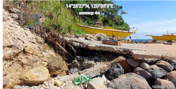
Collapse of the community boat landing areas due to high waves during the onset of typhoons
