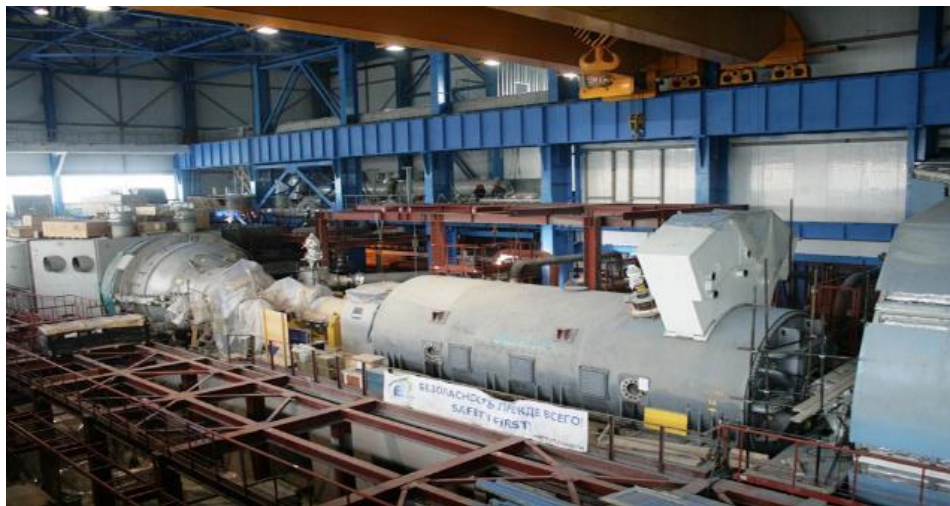
Figure 7: Sample of the Combined Cycle Gas Turbines with a capacity of 1600 MW
