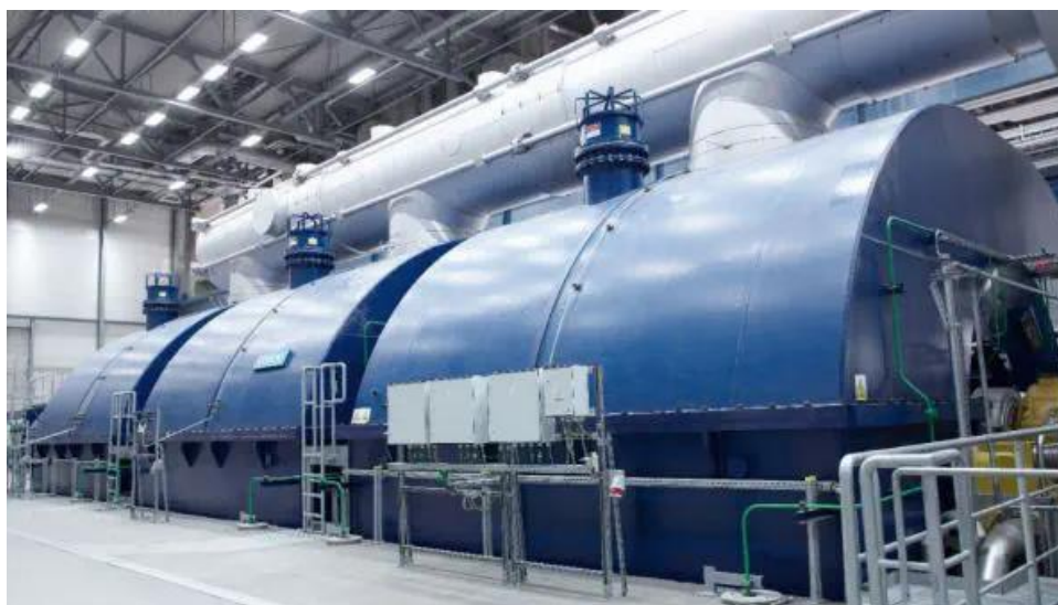
Figure 8: Sample of the Steam turbine "Siemens"
