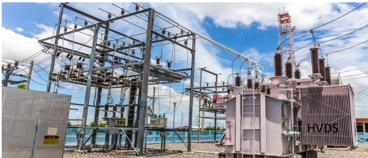
Figure 4-5: Typical HVDS &amp; Distribution lines
