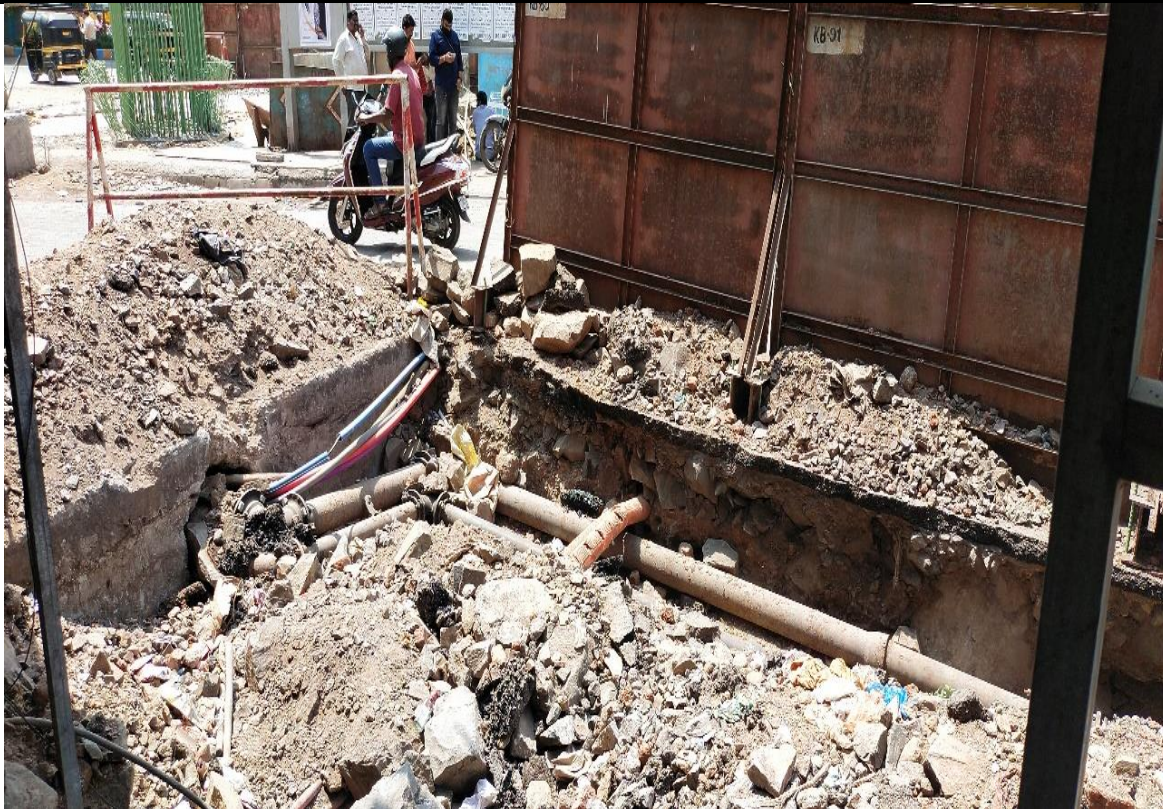
Figure 12: Poorly kept excavations risking worker and community safety
