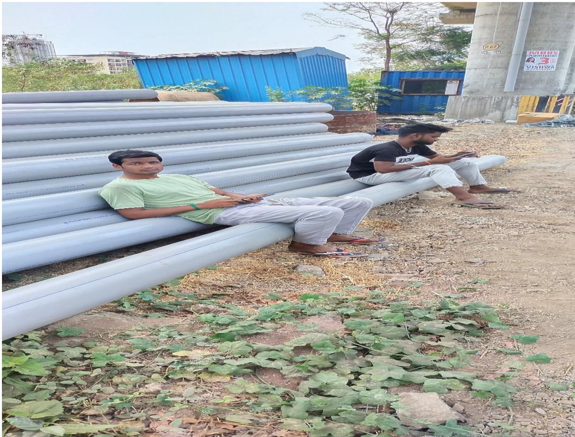
Figure 13: Sub-contractor's (vendor) workers with no PPE on site
