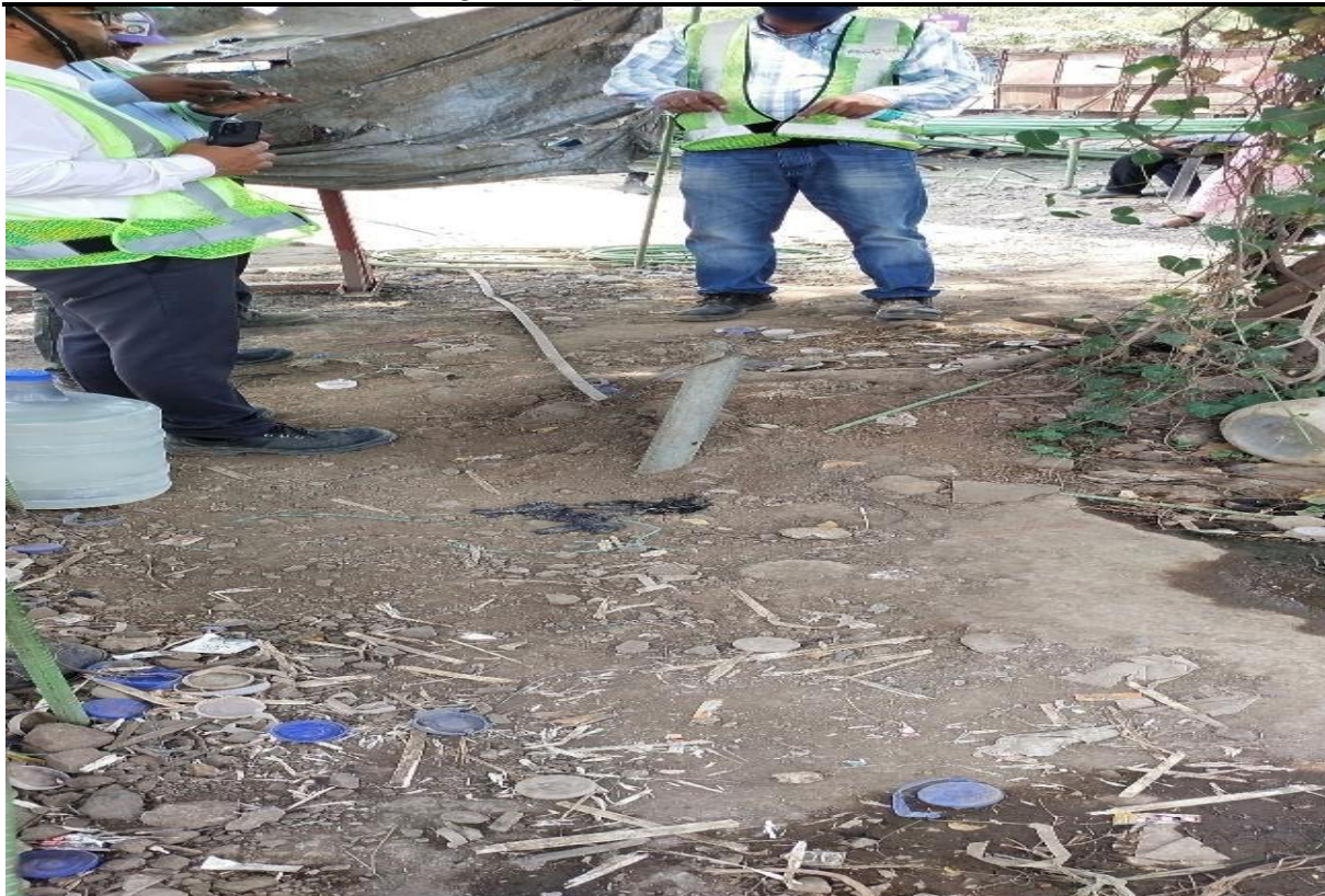
Figure 10: Poor earthing of machinery leading to trips and falls
