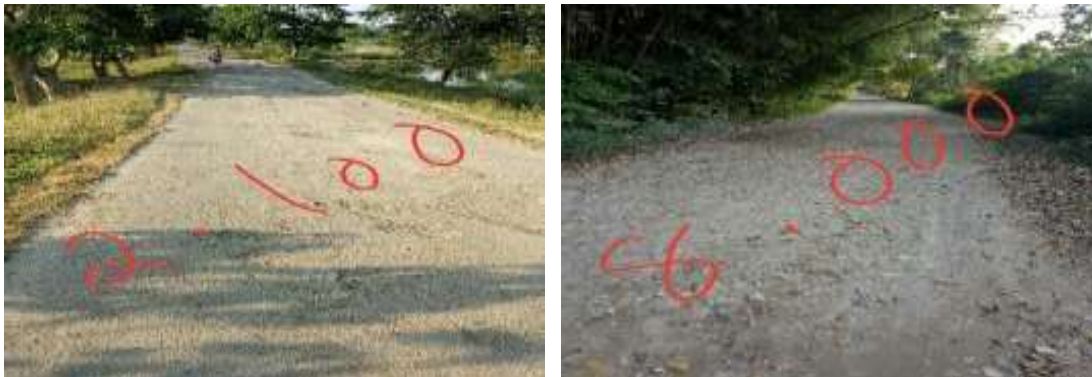
Figure 3.1 : Photographs of the pavement condition of the Project Road A-07
