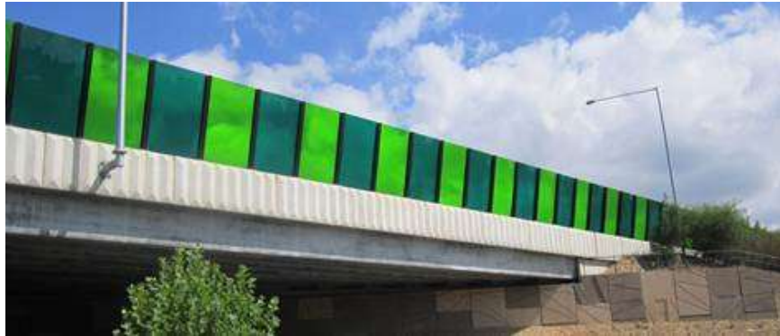
Figure 89: Bird anti-collision barrier
