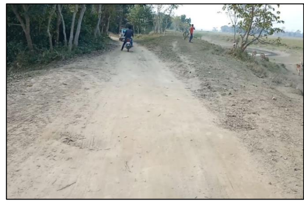
Exhibit-4: Road Condition
