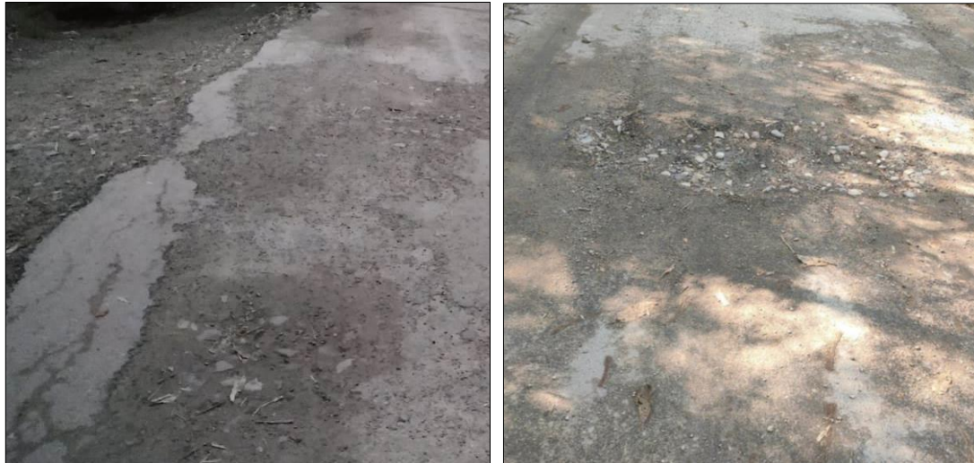
Figure 1- 3: Photo of highly distressed road along stretch
