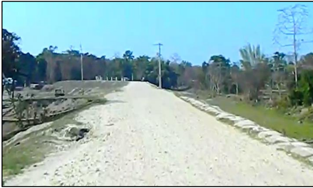
Exhibit-1: Road Condition
