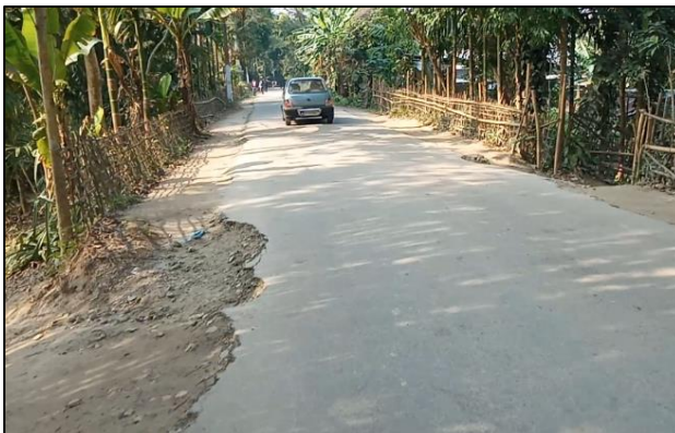
Exhibit-3: Road condition
