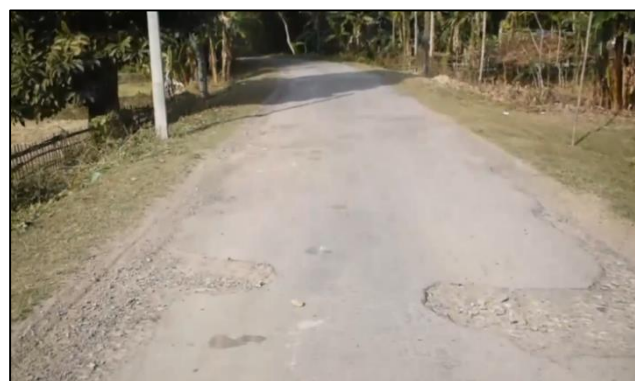
Exhibit-4: Road Condition
