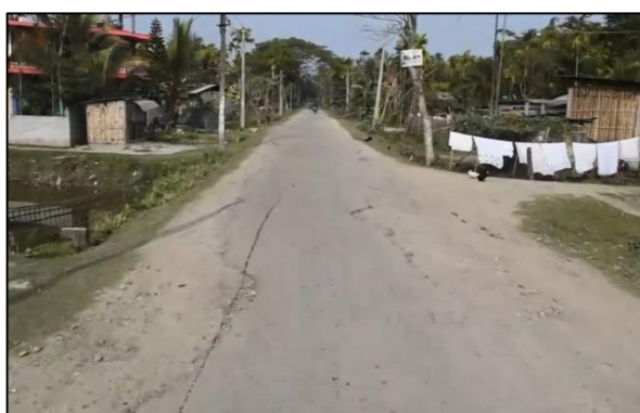
Exhibit-3: Road Condition
