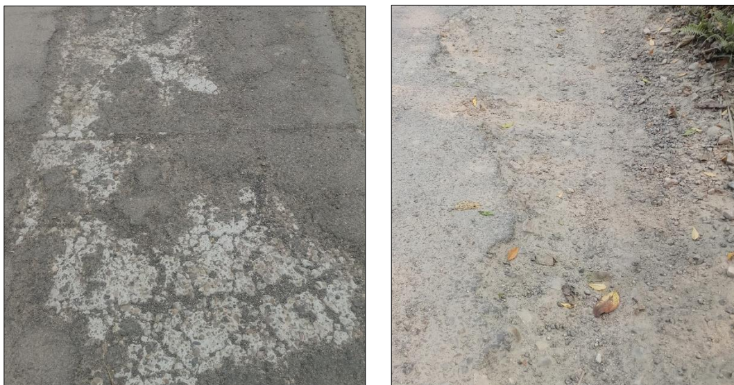
Figure 1- 3: Photo of highly distressed road along stretch
