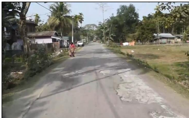
Exhibit-2: Road Condition
