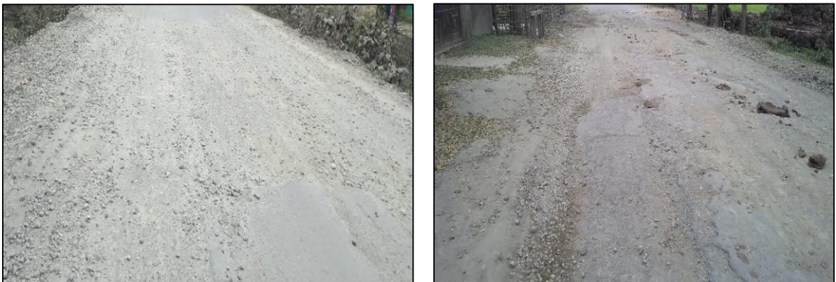
Figure 1- 3: Photo of highly distressed road along stretch
