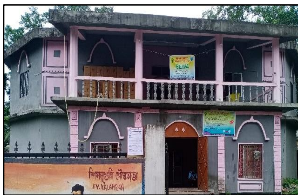
Affected boundary wall of the Govt. Office
