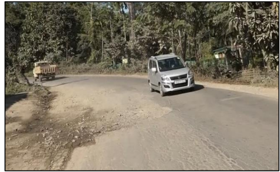
Exhibit-2: Road Condition at curve
