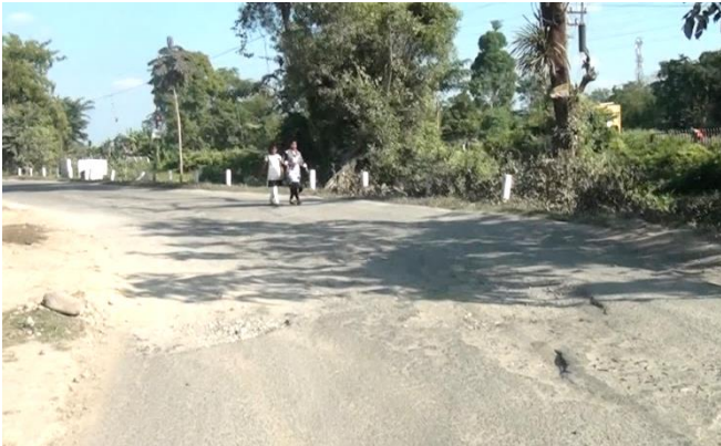
Exhibit-3: Road Condition
