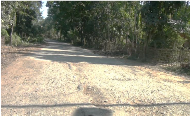
Exhibit-1: Road Condition
