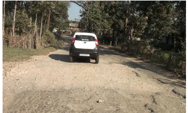
Exhibit-2: Road Condition
