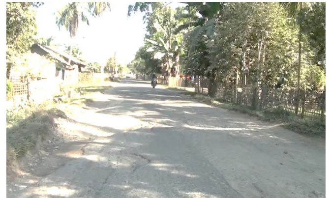
Exhibit-4: Road Condition
