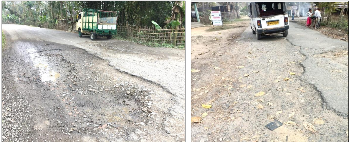
Figure 1- 3: Photo of highly distressed road along stretch
