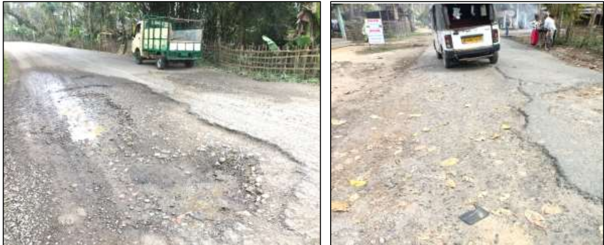
Figure 1- 3: Photo of highly distressed road along stretch
