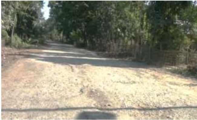
Exhibit-1: Road Condition
