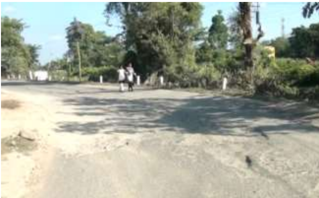
Exhibit-3: Road Condition
