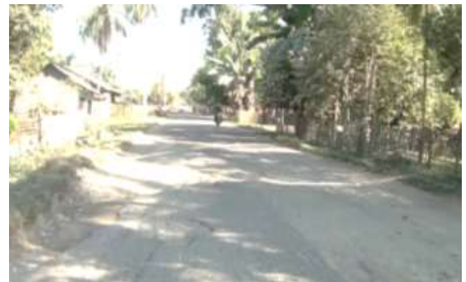
Exhibit-4: Road Condition
