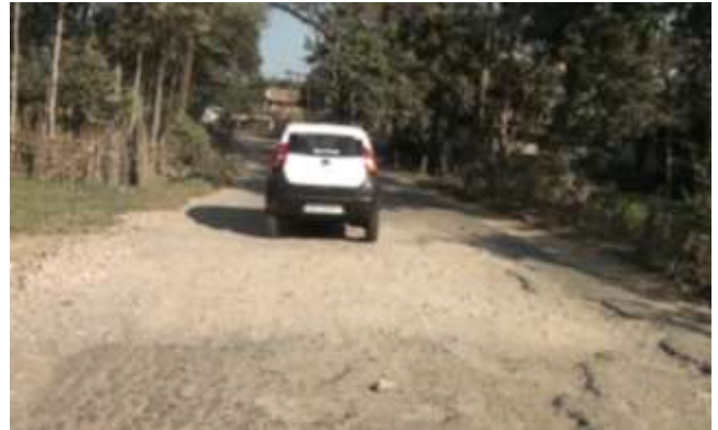
Exhibit-2: Road Condition
